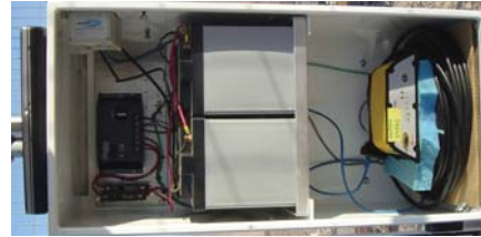
Figure 7. Interior of equipment box for station PCLL. Solar panel control unit and ethernet radio located above batteries, GPS receiver below.
