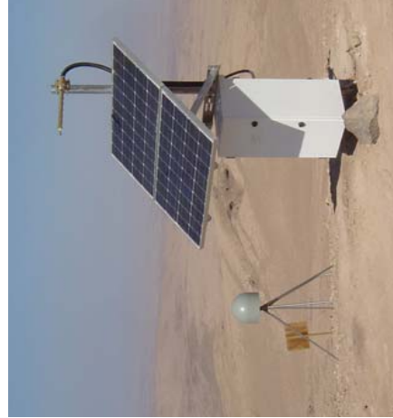
Figure 5. CAGA station KLN in northern Chile. Equipment box, solar panels, and ethernet link radio antenna in the foreground, GPS tripod and antenna in the background.
